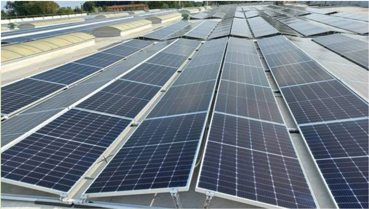
Solar power at Ingersoll Rand’s Vignate, Italy plant.
