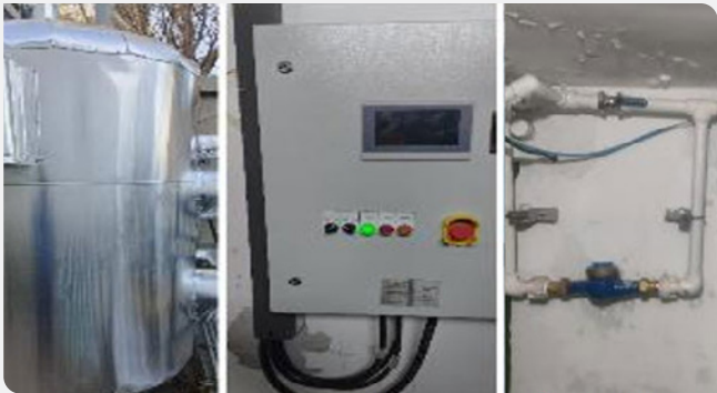
AFTER: By repurposing an old water tank to store condensate water, the system now pumps it to the workshop office building for reuse.
